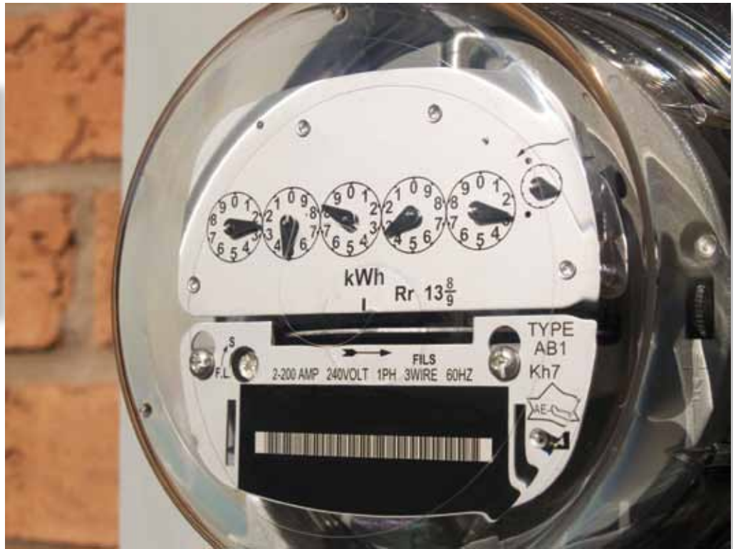
The electromechanical induction meter operates by counting the revolutions of an aluminum disc that rotates at a speed proportional to the power being consumed. This type of technology dates back to 1888, and these meters can only be read manually. Inaccuracies called "disc creep" can occur in these types of meters, causing inconsistencies in billing. ©iStockphoto.com/Trevor Fisher
